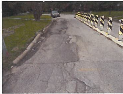
Localized Pavement Failure
